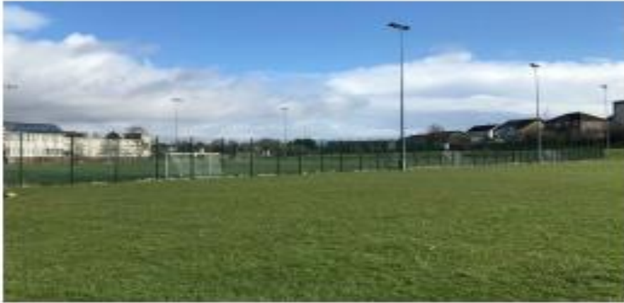
EXISTING ABACUS 15m HIGH LIGHTING COLUMNS
